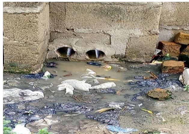
Figure 6. A paved house that discharges effluents through the fence into the street
