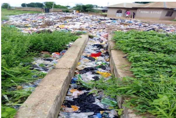
Figure 3. A drainage channel turned to refuse dump
