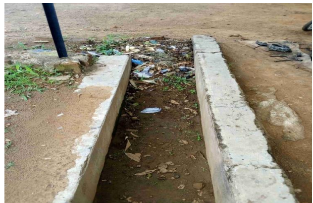
Figure 2. An unconnected drain
