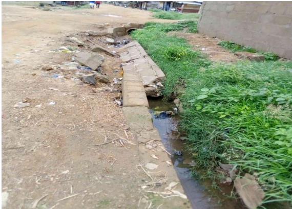
Figure 1. A failed drain due to poor construction work
